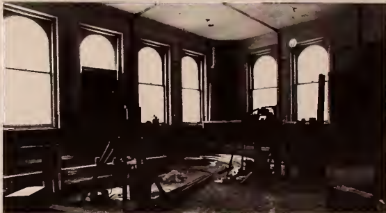
The tools of the trade ... Workers from the University's renovation crew will pick up where they left off in this photo, when they return for another day of refurbishing Weaver.
